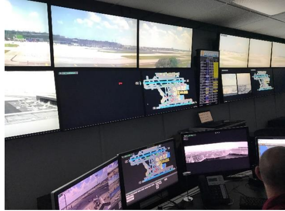
Virtual Ramp Control System at Ft. Lauderdale-Hollywood International Airport
